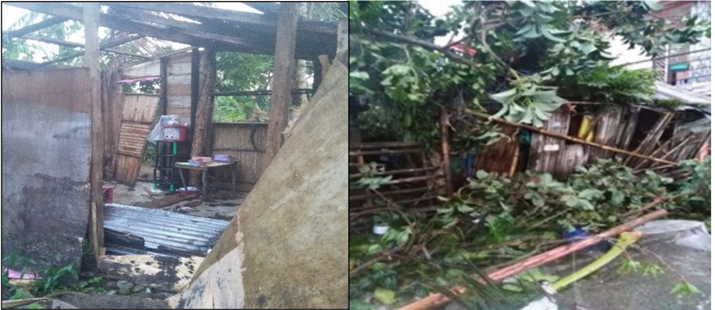
Figure 2: Housing Damages of Super Typhoon Rolly in Barangay Bogna (Left) and Barangay Buenavista (Right)
